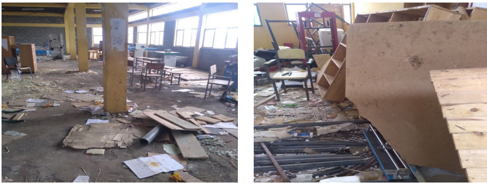
Figure 40. A photo showing the looted & damaged Amdework Technical & Vocational College workshop
