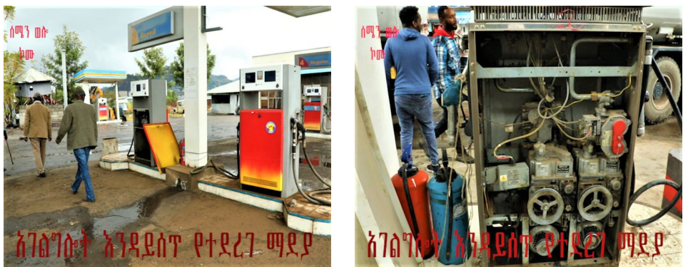
Figure 45. Gas stations that were made unavailable due to the destruction and looting of various parts by the invading forces (Gubalafto District)
