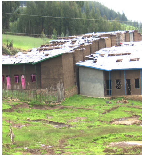
d) Houses damaged at laygaint woreda (Nefas Meucha)
