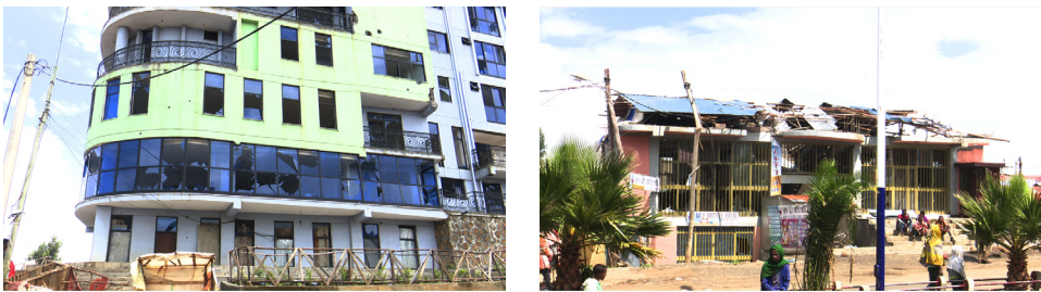
Figure 44. Business houses destroyed by the invading force Nefas Mewucha woreda)
