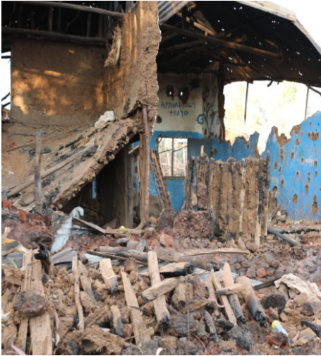
c) House Damage at Wadla woreda (Gashena)
